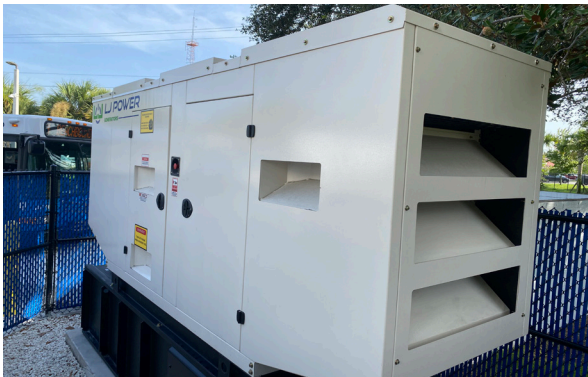
Pictured above is of a recent 2022 Brevard County Space Coast Area Transit Generator replacement. The project’s electrical design was for a 100 kW generator and underground feeder. Moncef played a key role for the success of this project.
