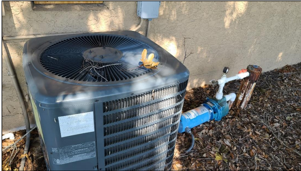
VIEW OF HVAC
