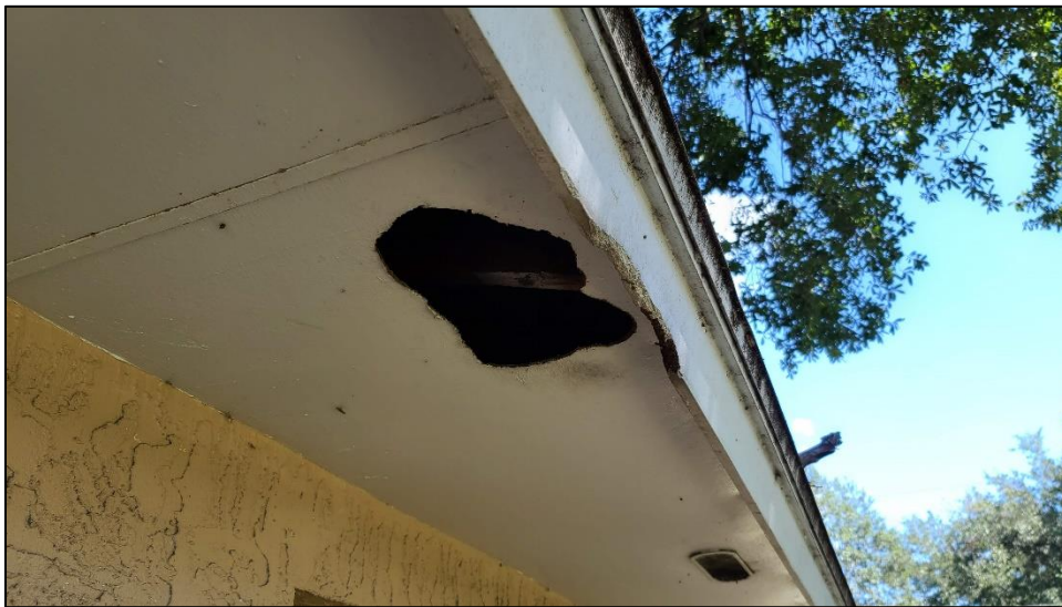
VIEW OF SOFFIT HOLE
