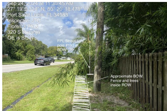
Figure 9 – FPL Pole Sidewalk Conflict
