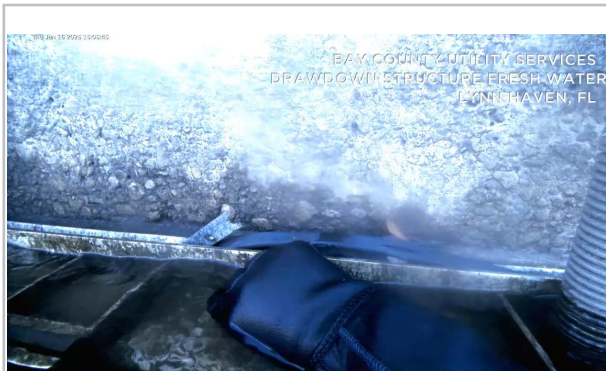
Deformed Gasket/ Missing Hardware (Gate #2)
