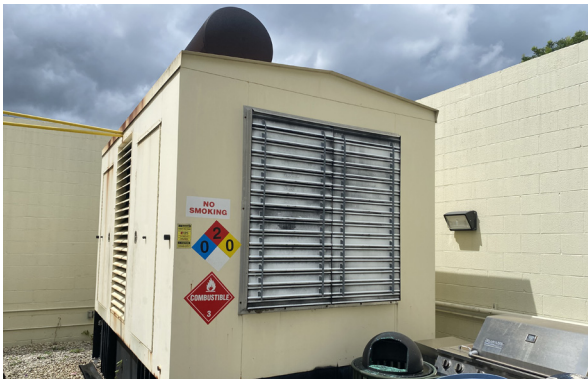
Pictured above is of a recent 2024 City of Port St Lucie, Generator Building B replacement. The project 's electrical design was for a 1,000 kW generator and underground feeder. John plays a key role for the success of this project.
