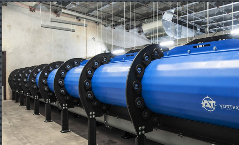
Action Target Containment System *Note ceiling "height"
