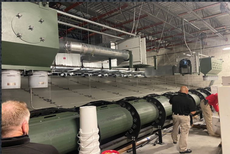
Palm Beach Gardens Firearms Range Bullet Trap Containment System **Note ceiling height**
