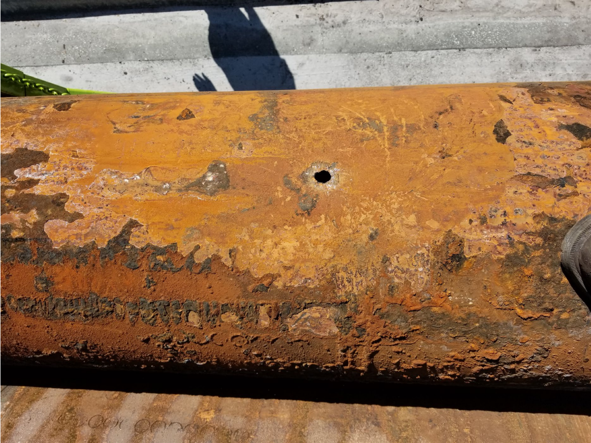
The tubing failure due to corrosion at the JEA Water Treatment Plant IW-1.
