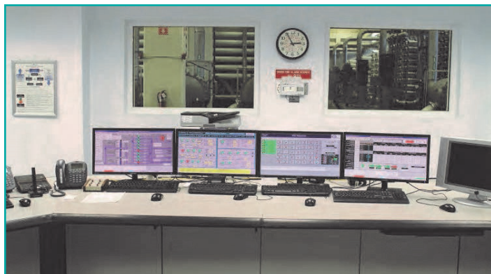
Figure 11. AECOM has designed instrumentation and control and Supervisory Control and Data Acquisition systems on many projects, including several for Collier County and the City of Fort Myers.
