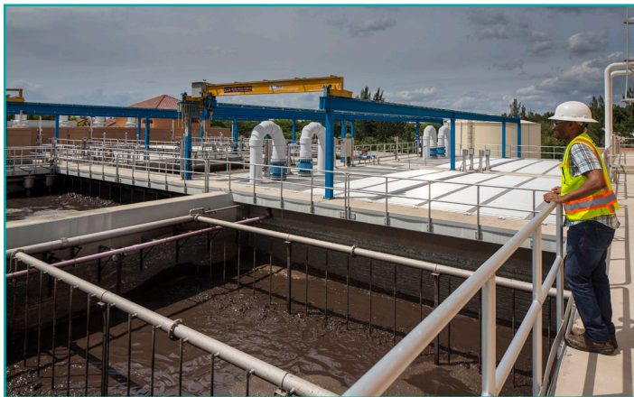
Figure 4. AECOM provided facilities planning and was the design-builder for the Town of Davie's new water treatment and water reclamation facilities.
