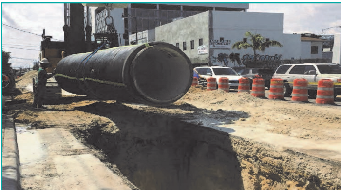
Figure 8. The City of Miami Beach was concerned that failure could prove catastrophic to the Miami Beach community, causing discharge of millions of gallons of raw sewerage that can affect safety, human health, coastal environment, and local business operations. To mitigate the risks, the City contracted with AECOM to fast track the development and installation of a new 54-inch redundant pipeline that achieves the redundancy objective and utilizing trenchless approaches.
