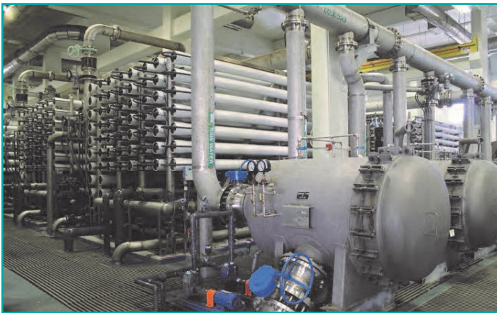
Figure 2. AECOM is the original designer of Collier County’s NCRWTP and was responsible for the addition of RO treatment at the SCRWTP.
