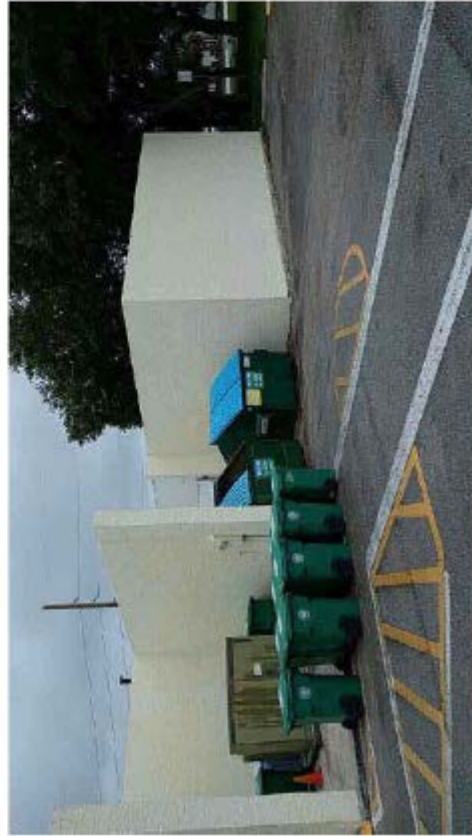
#3 - Transformer & FPL Meter & dumpster area
