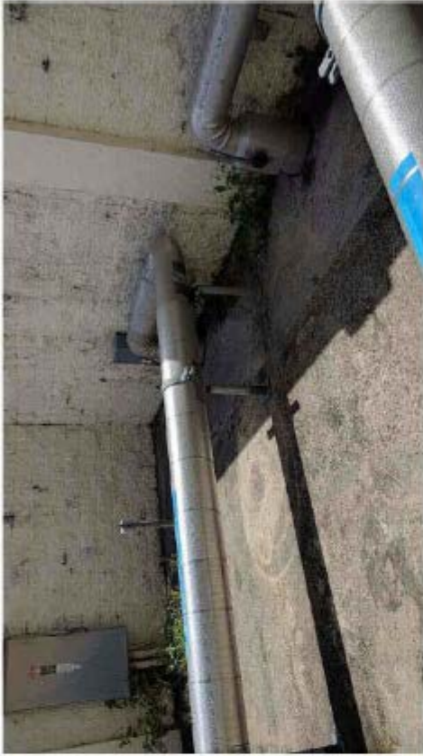
#10 - Chiller yard at South wall
