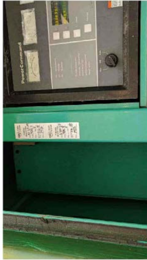
#15 - Generator controls close up
