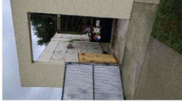
#4 - Access Gate to Generator
