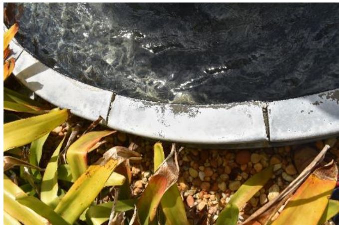
Figure 77. Failed mortar joints on the base of the fountain. The black liner is visible beneath the water and the coating on the perimeter is beginning to deteriorate on the inner edge (Photo by EverGreene, October 2022).
