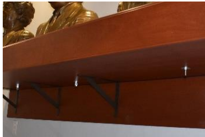
Figure 34. Missing bolt from beneath the right most bust (Photo by EverGreene, October 2022).
