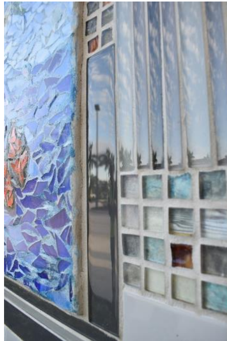
Figure 67. Cracking of mosaic joint along the exterior right side (Photo by EverGreene, October 2022).
