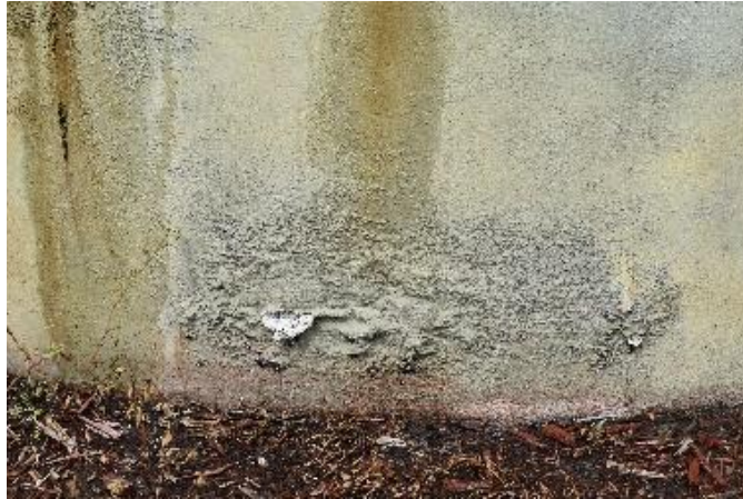
Figure 8. Efflorescence beneath the paint coating on the concrete base with visible staining and dampness seeping in the area (Photo by EverGreene, October 2022).
