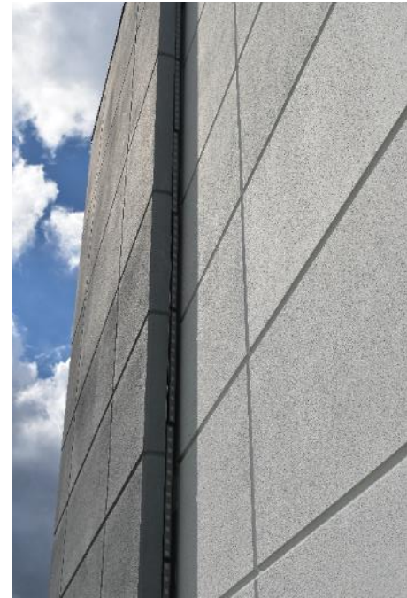
Figure 107. Dislocated light strips 5, 6, and 8 of East light assembly #1 (Photo by EverGreene, October 2022).
