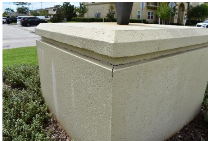
Figure 27. Horizontal joint failing on the concrete base. There is a portion of the network of cracks visible on the right face of the base and salt staining on the left face (Photo by EverGreene, October 2022).
