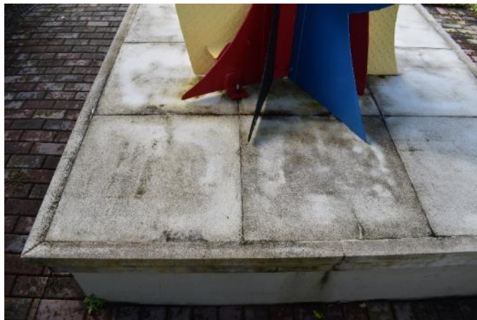
Figure 115. Atmospheric and biological staining on the top face of the concrete base (Photo by EverGreene, October 2022).
