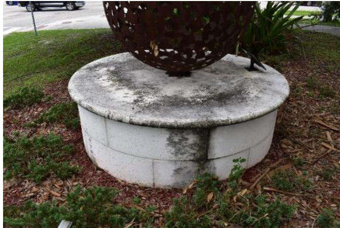
Figure 60. Atmospheric and biological staining on the surface of the stone base (Photo by EverGreene, October 2022).
