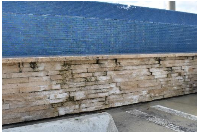
Figure 100. Detail image of stones on the northwest elevation of the fountain base. There is biological staining and growth in between the stones and on the stone surfaces, as well as efflorescence and calcium deposits (Photo by EverGreene, October 2022).
