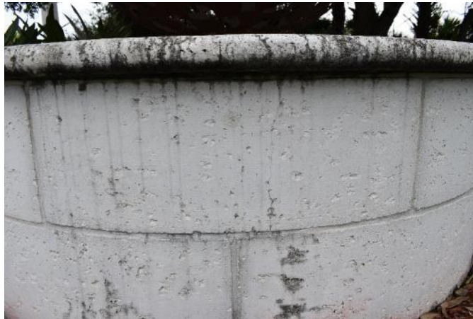
Figure 61. Crack through the stone base (Photo by EverGreene, October 2022).
