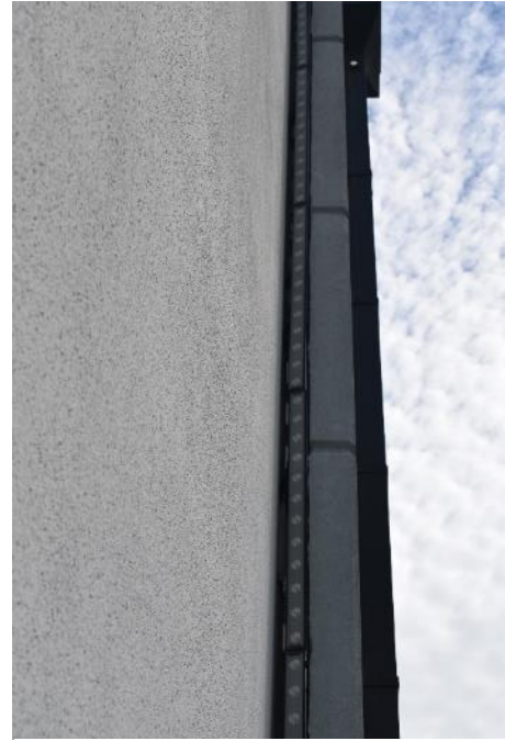
Figure 105. Dislocated light strip 7 of South light assembly #1 (Photo by EverGreene, October 2022).
