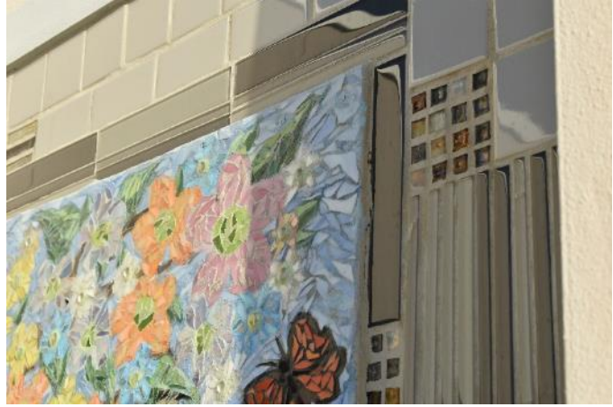
Figure 74. Cracking of mosaic joint along the exterior right side (Photo by EverGreene, October 2022).
