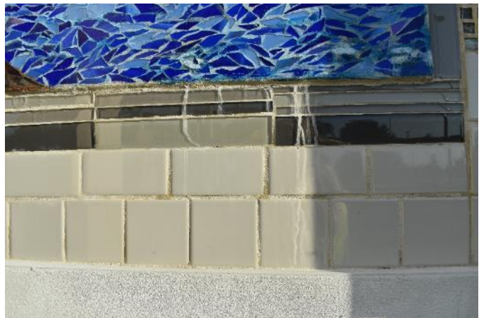
Figure 75. Calcite and salt residue seeping from the crack in the bottom exterior mosaic joint onto the surface of the perimetral tiles (Photo by EverGreene, October 2022).
