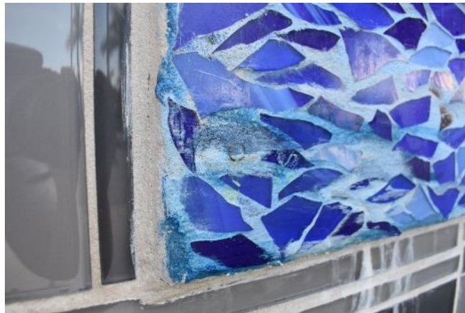
Figure 64. Evidence of ferrous mounting hardware exposed by erosion of blue grout (Photo by EverGreene, October 2022).
