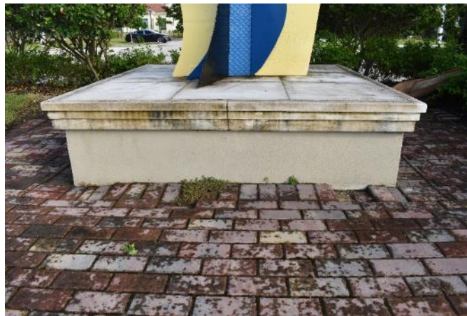
Figure 117. Biological growth in the grout of the cornice on the concrete base (Photo by EverGreene, October 2022).
