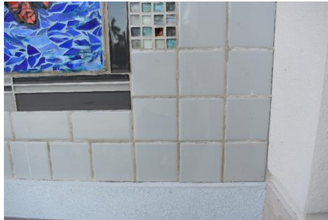
Figure 68. Discoloration/darkening of perimetral tile grout (Photo by EverGreene, October 2022).
