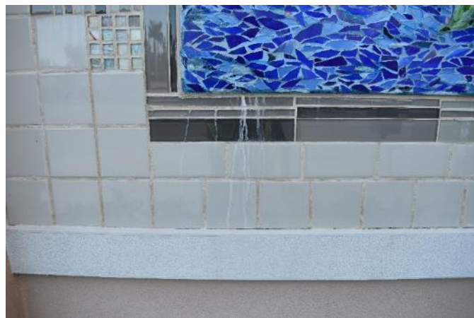
Figure 69. Calcite and salt residue seeping from the crack in the bottom exterior mosaic joint onto the surface of the perimetral tiles (Photo by EverGreene, October 2022).
