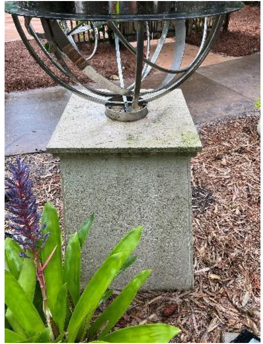
Figure 23. Corrosion at the base of the sphere and biological growth on concrete base (Photo by EverGreene, October 2022).
