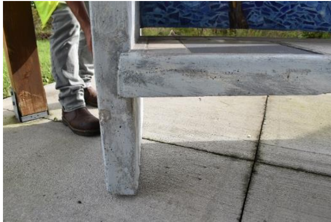
Figure 41. Minor material loss in the front left leg of the bench (Photo by EverGreene, October 2022).
