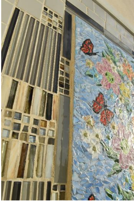
Figure 73. Cracking of mosaic joint along the exterior left side (Photo by EverGreene, October 2022).
