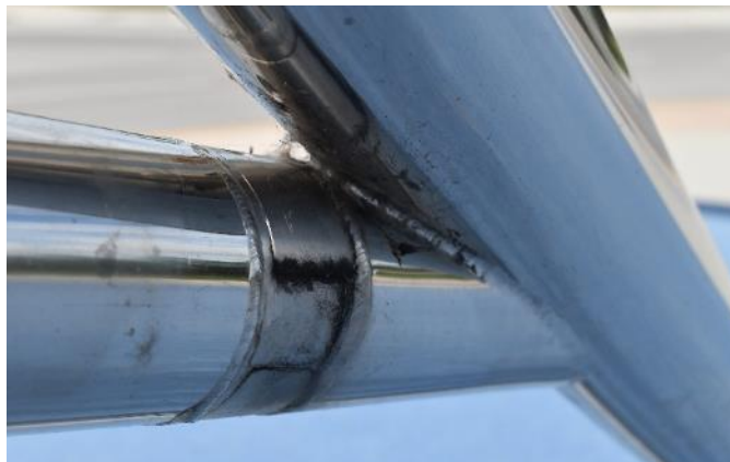
Figure 124. Corrosion at the joint of two poles (Photo by EverGreene, October 2022).
