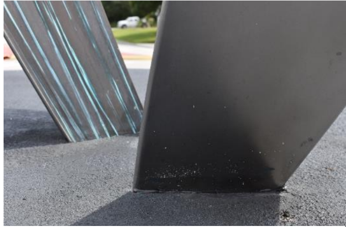
Figure 120. Sealant failure at the base of one of the metal uprights (Photo by EverGreene, October 2022).
