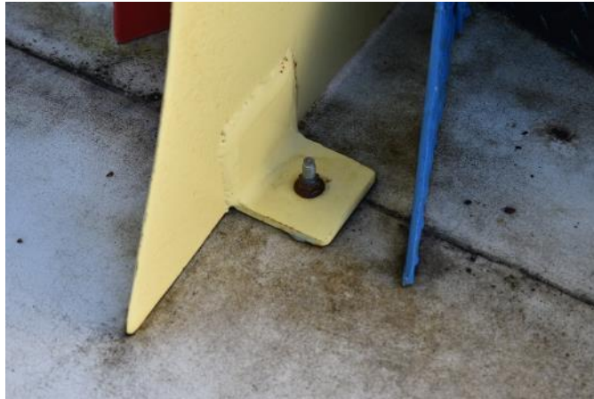
Figure 114. Ferrous mounting hardware on the base of the sculpture that is corroding (Photo by EverGreene, October 2022).
