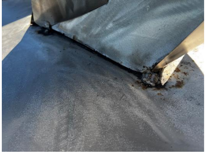
Figure 86. Metal corrosion on the surface of the base of the sculpture, resulting from losses in the clear coat (Photo by EverGreene, October 2022).
