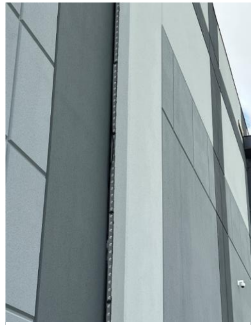
Figure 111. Exposed cable on light strip 3 of North light assembly #1 (Photo by EverGreene, October 2022).
