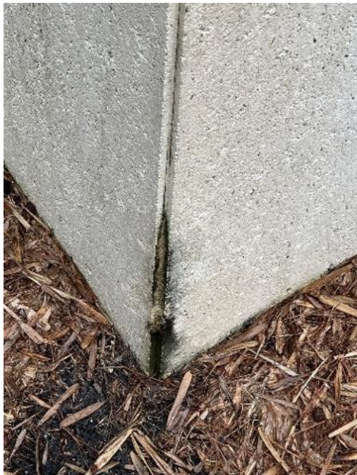
Figure 24. Vertical joint with biological growth and residual staining (Photo by EverGreene, October 2022).
