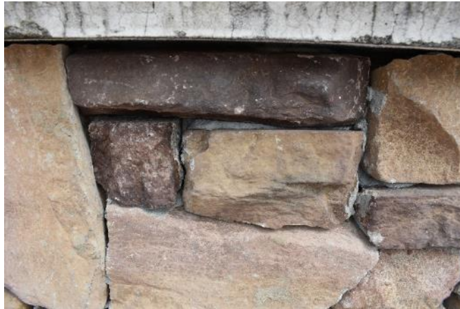
Figure 32. Failing mortar joints on the vertical face of the stone base (Photo by EverGreene, October 2022).
