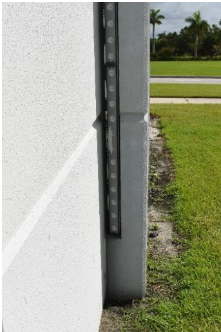
Figure 106. Paint or epoxy residue on light strip 1 of South light assembly #3 (Photo by EverGreene, October 2022).
