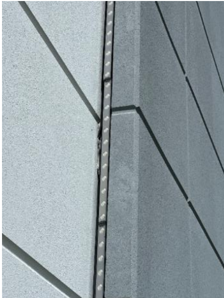
Figure 108. Possibly broken or light strip 4 of East light assembly #4 (Photo by EverGreene, October 2022).
