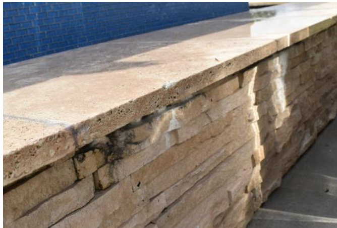
Figure 102. Detail image of efflorescence and calcium deposits on the northwest elevation of the fountain basin (Photo by EverGreene, October 2022).
