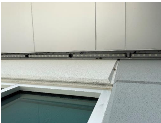
Figure 110. Insects nesting in the Northeast horizontal light assembly #1 (Photo by EverGreene, October 2022).
