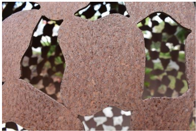
Figure 58. Detail image of the surface of the exterior of the sphere. The metal is completely corroded across the surface (Photo by EverGreene, October 2022).
