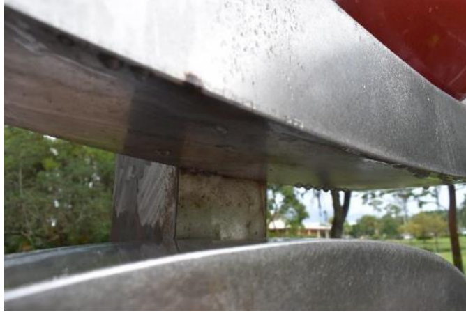
Figure 21. Ferrous staining on surface of the reverse of the textured cube between the two rectangular elements (Photo by EverGreene, October 2022).
