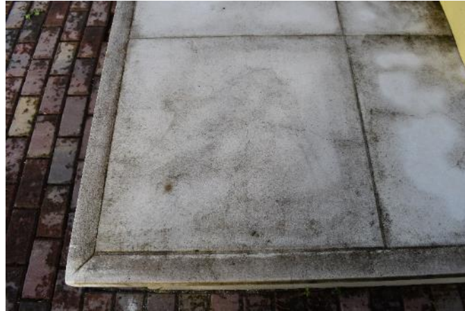
Figure 116. Crack network on the top face of the concrete base (Photo by EverGreene, October 2022).
