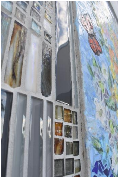
Figure 66. Cracking of mosaic joint along the exterior left side (Photo by EverGreene, October 2022).
