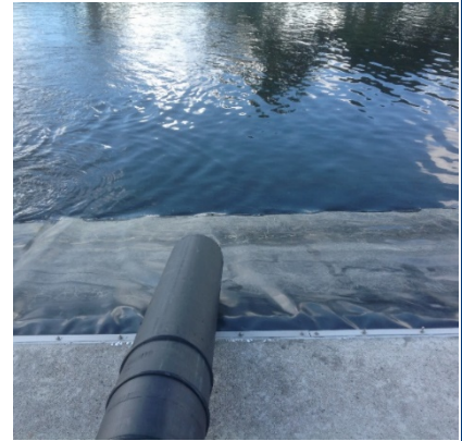
SLWSD WWTF Reclaimed Water - ROWTP Concentrate Blending Line
