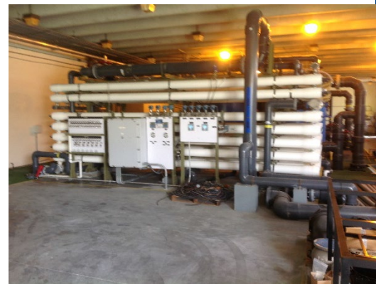
SLWSD ROWTP Skid
