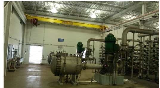
Melbourne ROWTF Feed Pump System improved by Jacobs
