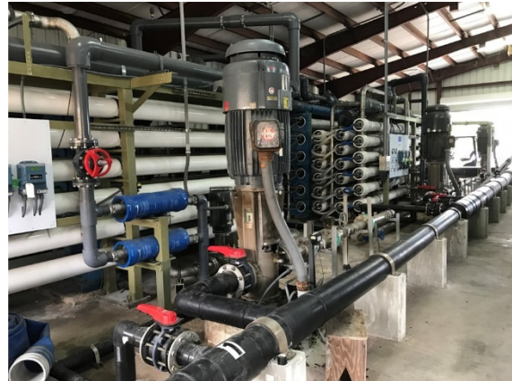
North Key Largo Reclaimed Water System RO Membrane Treatment Skids
