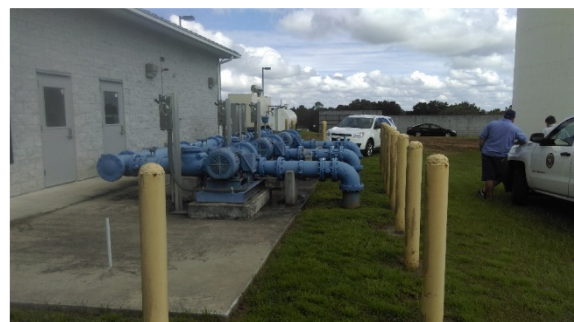
Dade City Orange Valley Booster Pump Station Site
