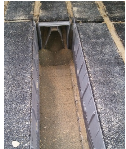
One of projects ongoing is the refurbishment of lime softening dual-media filters. The Leopold underdrains were failing, and the filter media had to be replaced. The work is currently being performed successfully one filter at a time.
