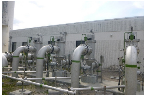
Sand strainers to remove solids loading from cartridge filters and provide additional protection for the membranes
