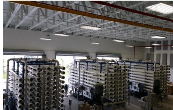
Three 2.25 mgd Reverse Osmosis skids for hardness and colour removal from the Biscayne Aquifer Source Water
