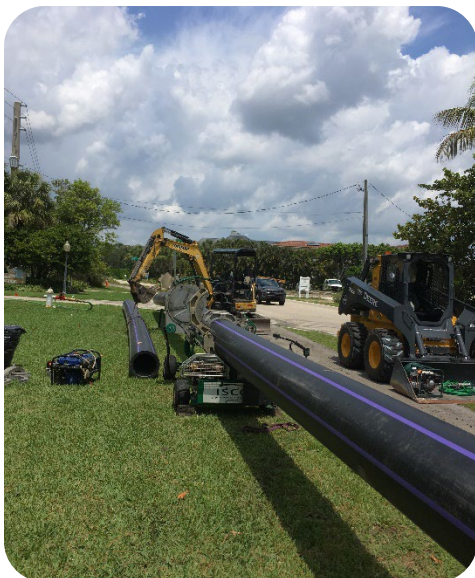
HCE will ensure that utility improvement projects are completed on time and within budget
