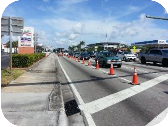
HCE has extensive experience with utility improvement projects constructed in crowded right-of-ways
