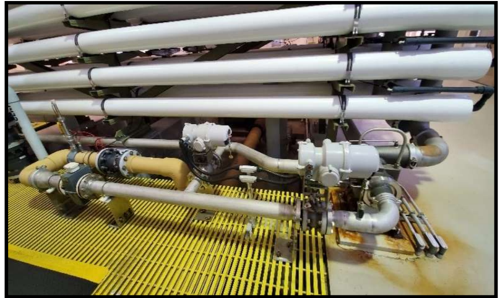
Concentrate Piping and ERDs. Skids 1-3 device (Left). Skids 4-10 device (Right)
