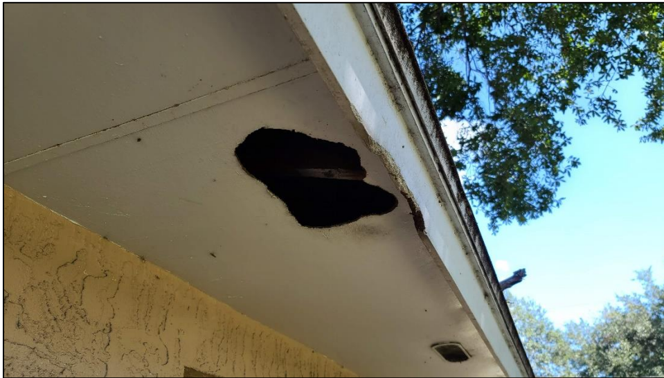
VIEW OF SOFFIT HOLE
