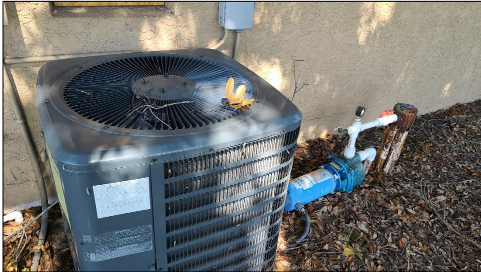
VIEW OF HVAC
